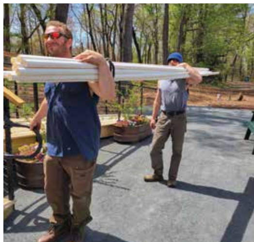
Sam Cashdollar and Jeremy Cole carrying irrigation pipe to install by restroom area.
